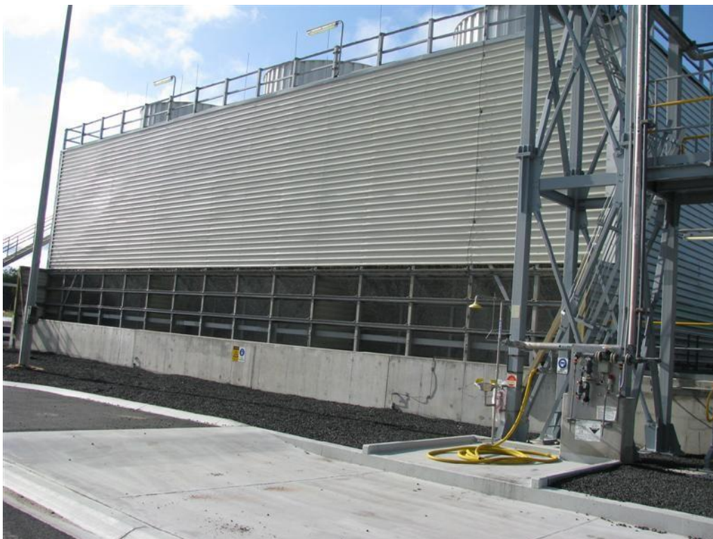
Figure 1: ACW Cooling Tower
