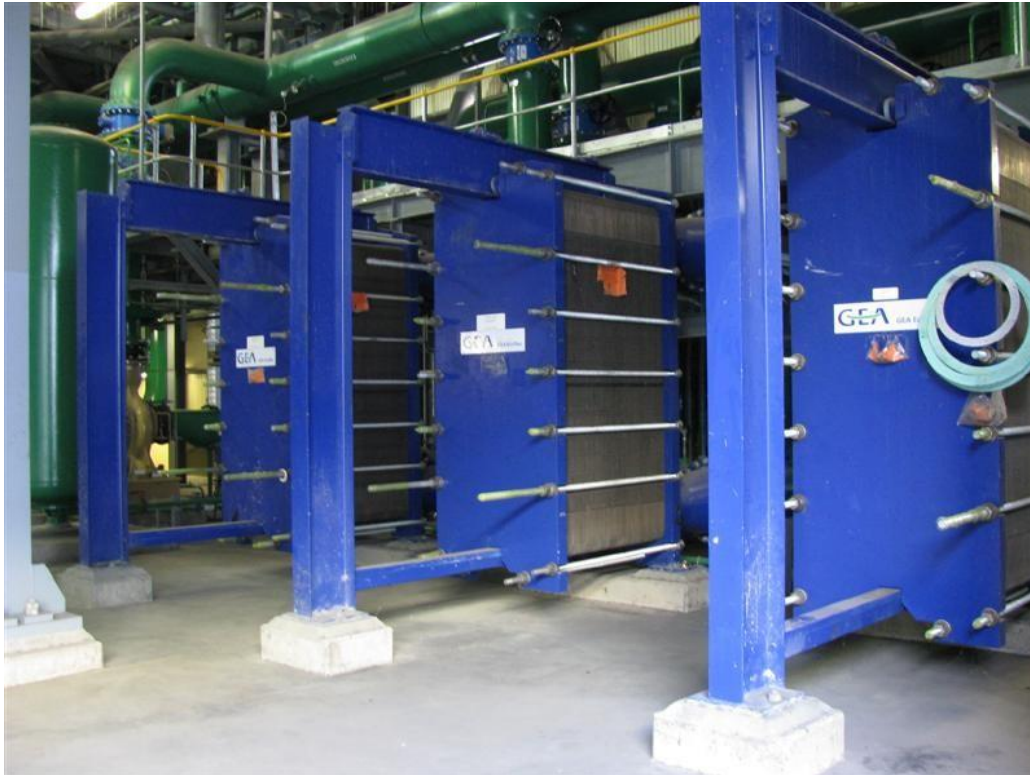
Figure 2; ACW/CCW Heat Exchangers
