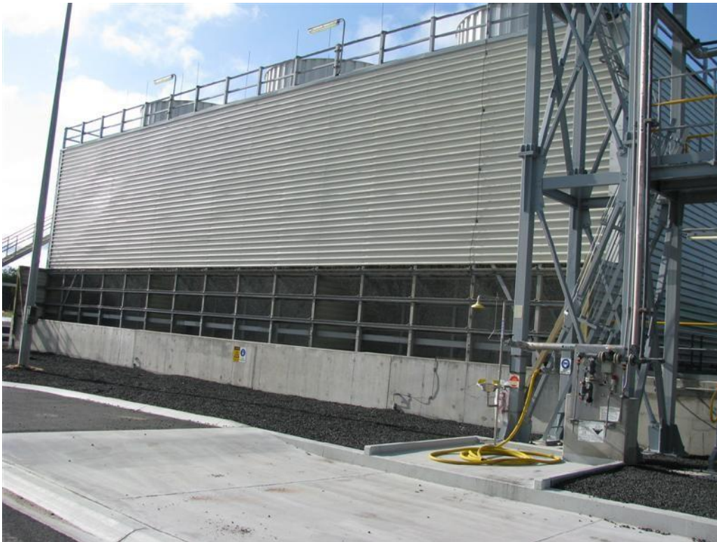
Figure 1: ACW Cooling Tower
