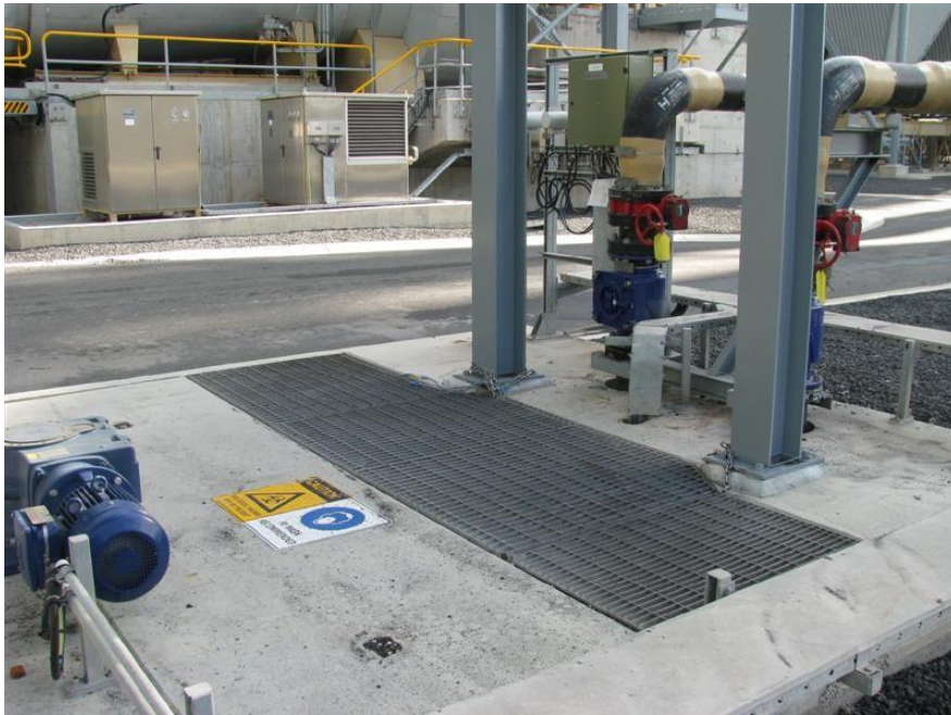
Figure 5 SCC cooling water pump pit
