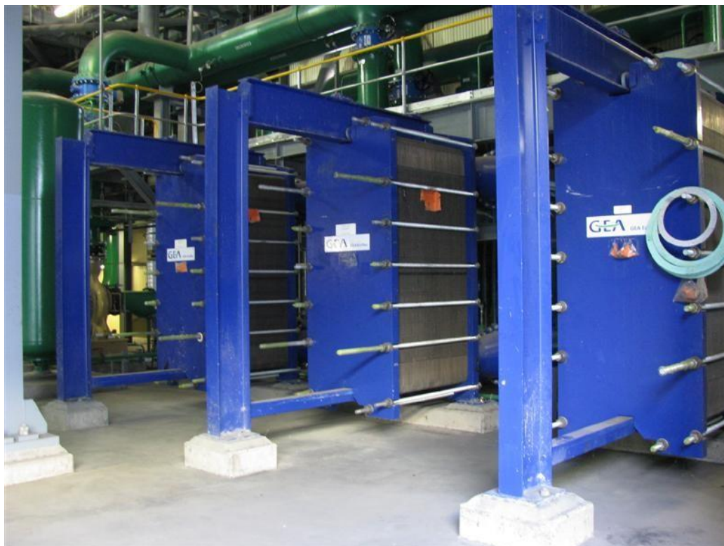
Figure 2; ACW/CCW Heat Exchangers
