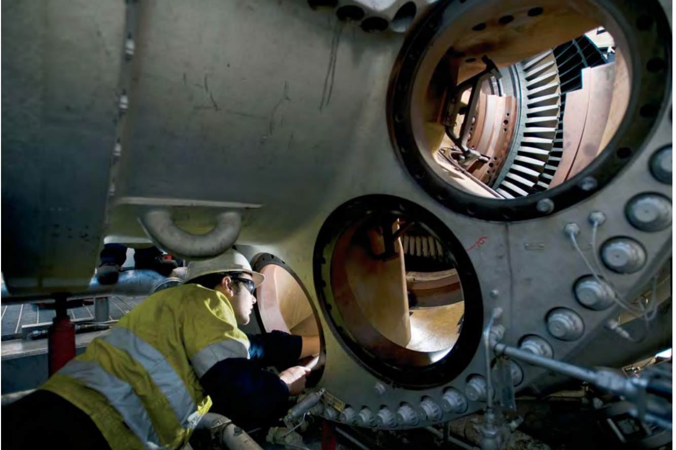
Inspection of the Mica Creek Power Station Unit A6 turbine during this year's planned overhaul
