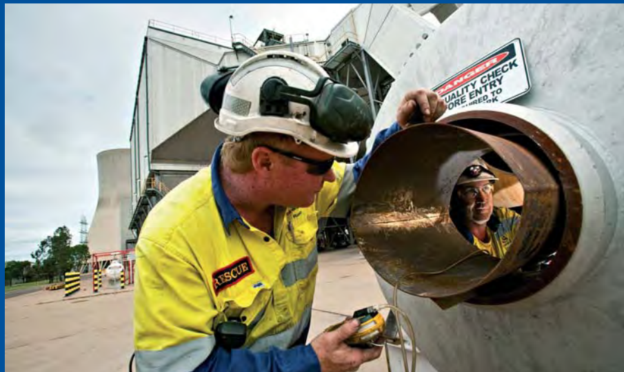
Shane McGovern and Dan van Haeran, Emergency Response Team members, test the new process in the mock-up heater
